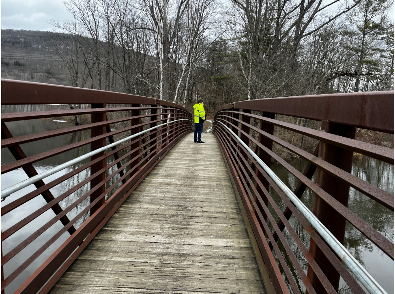
Pedestrian bridge crossing Housatonic River in Reach 6, approximately 3,000 feet north of the Upland Disposal Facility.
